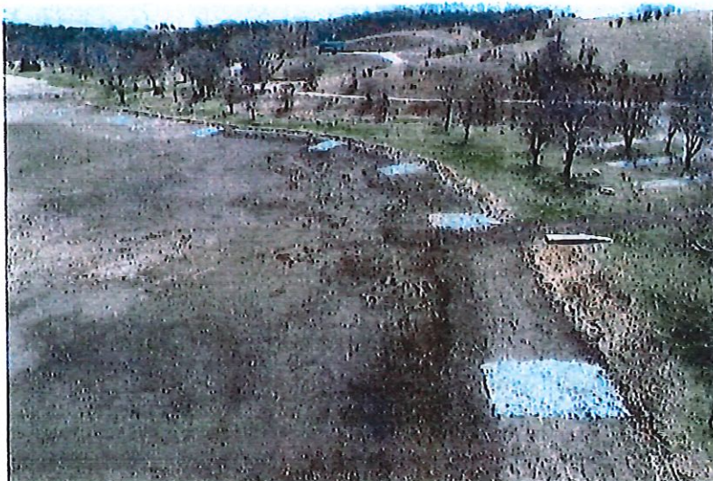
Figure 8. Gravel Spawning Bed. A combination of small riprap (Class A) and crushed limestone are placed in lake footprint adjacent to shoreline to block aquatic vegetation and provide fish habitat (photo from Summit Lake during lake drawdown).
