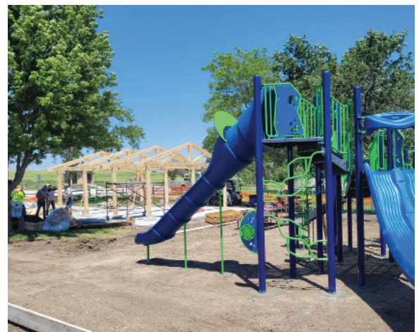
New playground and picnic equipment was installed at Smith Creek Recreation Area in the summer of 2024.
